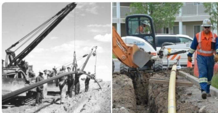
Throughout the years, the technology we use in our day-to-day operations has changed considerably - to create efficiency, improve safety, and to prevent infrastructure damage. Left: A steel natural gas transmission pipe being lowered by a crane mounted on a Caterpillar in 1952. Right: A backhoe and a Bobcat excavator dig to install a 6-inch steel natural gas line in 2015.
